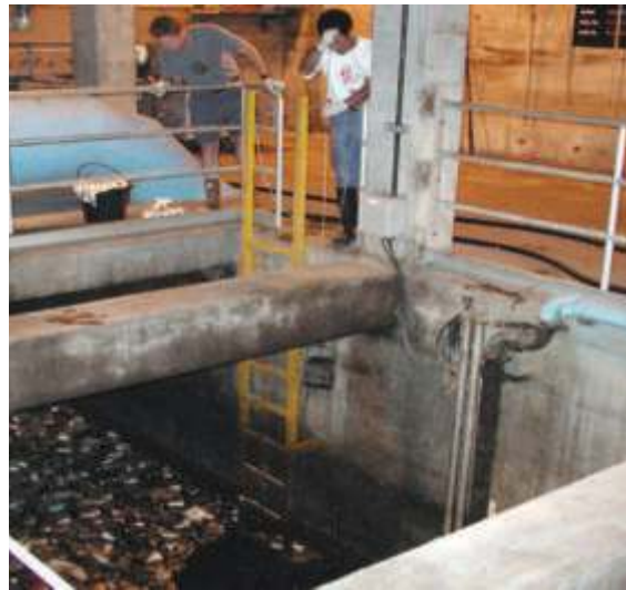
Inside the Ettie Street Pump Station. Photo courtesy of Applied Marine Sciences.
