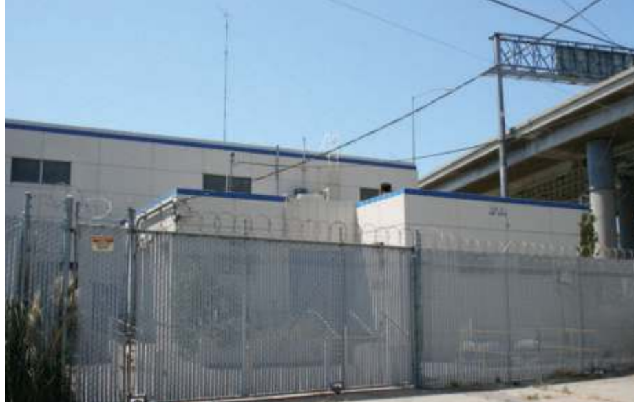
The Ettie Street Pump Station.
